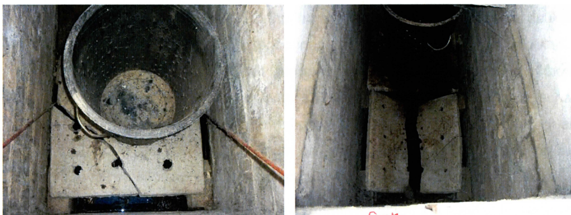
Figure 5: Broken drying plates in Grundorn and Nico Noord
